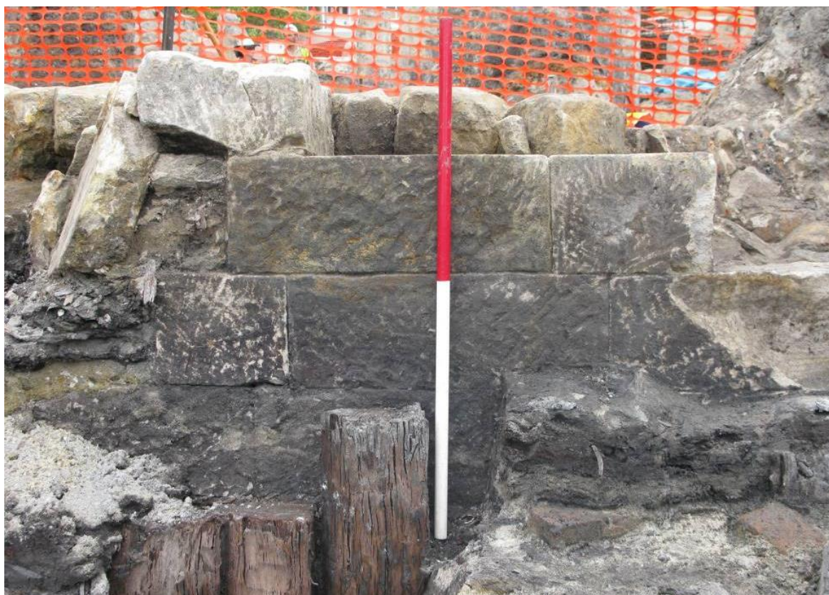
Figure 3.5.20: Detail showing the stones facing the harbour neatly cut and with chisel mark surfacing on the face. View to south. Scale 1m.
