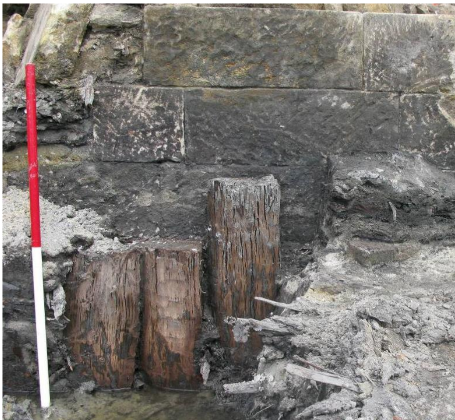
Figure 3.5.13: Detail of the top of the formwork (8460) and the stone wall behind. The right of the frame shows the amount of harbour deposits and accumulation against the wall. View to the south. Scale 1m.
